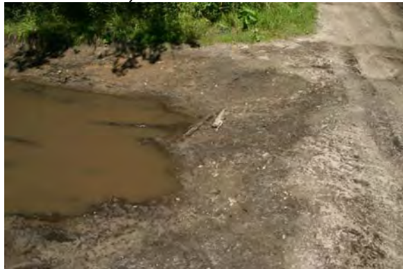
Plate 42: Flooded roadway with Corduroy Road eroded from the roadway..
